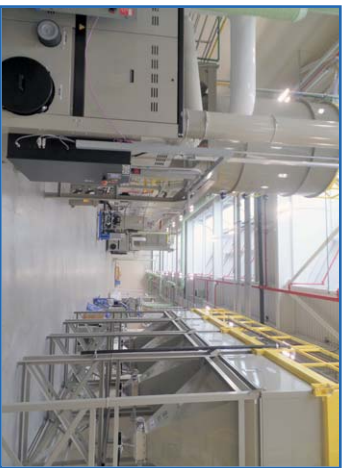
VIEW OF CONAIR RESIN DRYING AND HANDLING SYSTEMS
