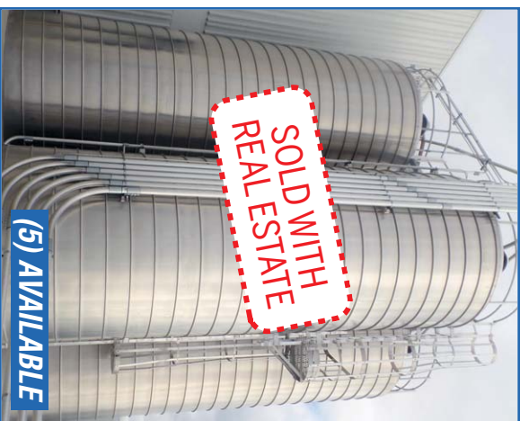
PARTIAL VIEW OF S/S SILOS
