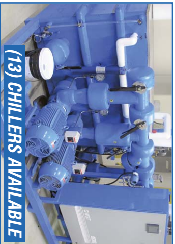
PARTIAL VIEW OF BERG CHILLER SYSTEMS
