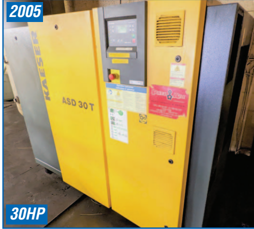
2005 KAESER ASD 30T COMPRESSOR
